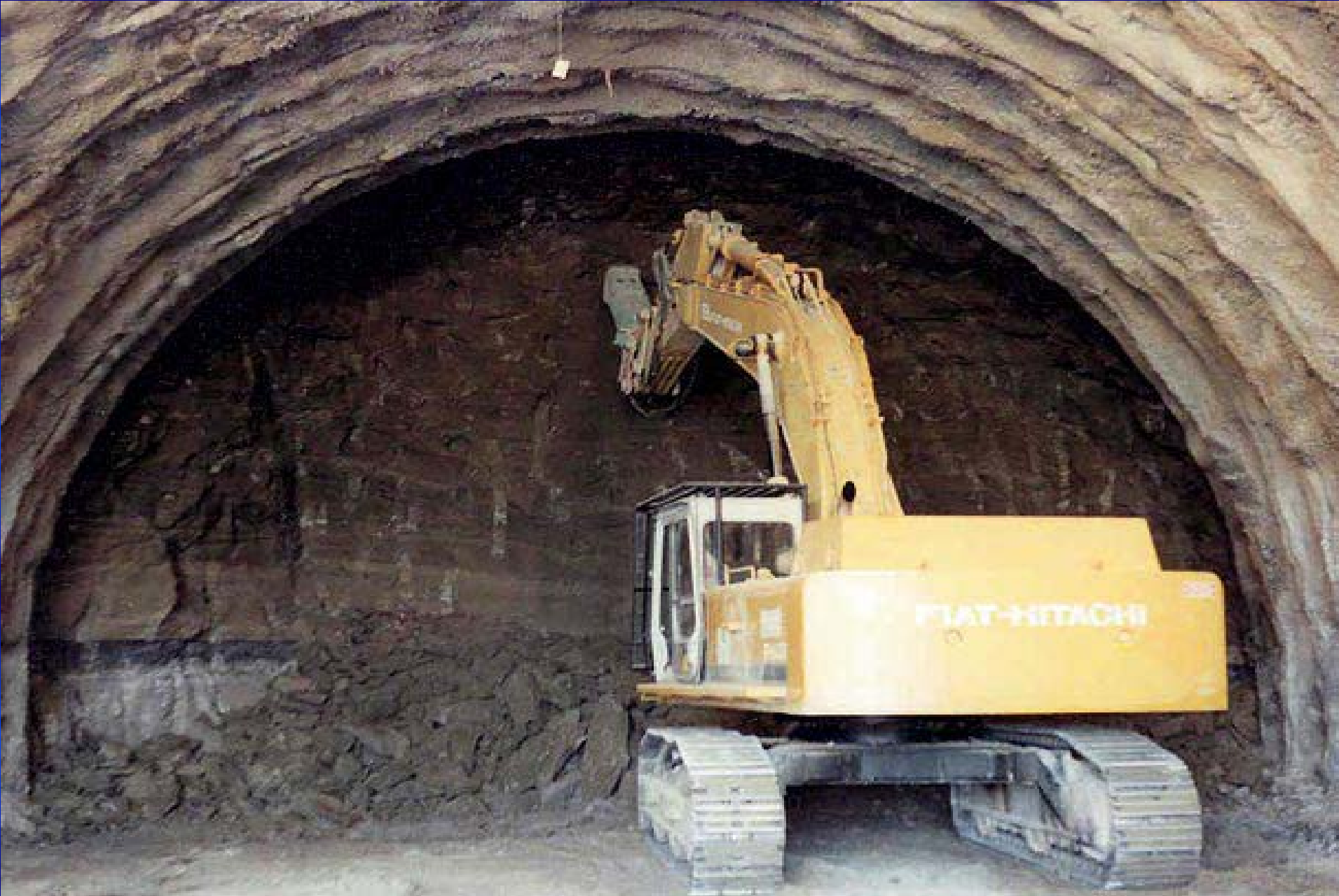
Macchia Piana Tunnel. Face reinforced with fibre glass structural elements. Ground: tuff, Overburden: ~ 3 m. [Lunardi Proyect]
