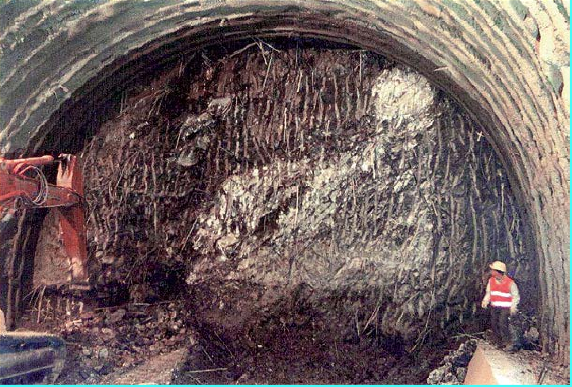
Colle Pece Tunnel. Face reinforced with fibre glass structural elements. Ground: scaly clays. Overburden: ~ 25 m [Lunardi Proyect]
